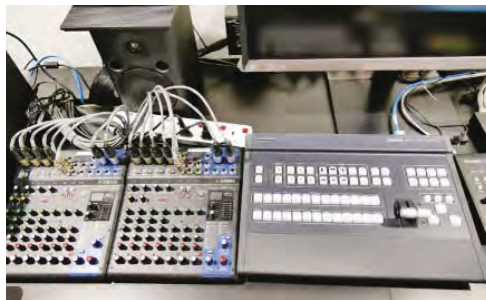
Yamaha MG10XU analogue mixers provide individual audio control in each ballroom division
