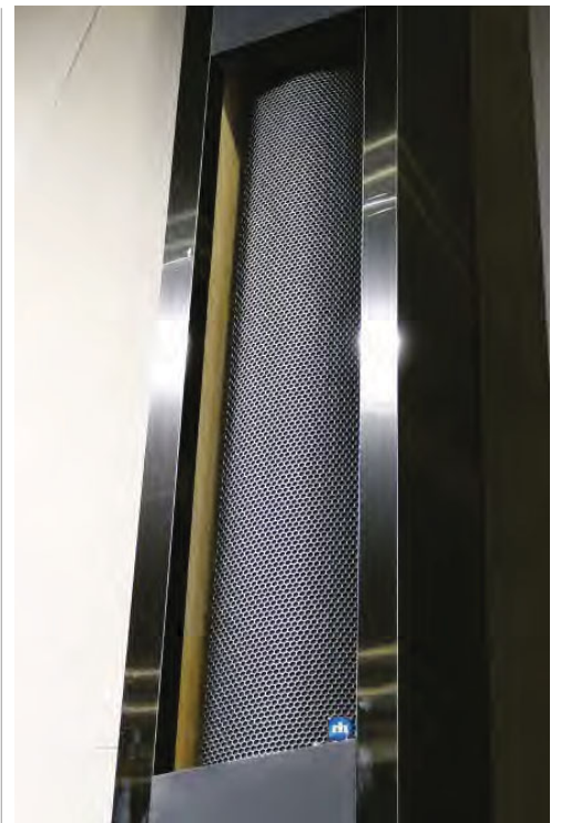
Renkus-Heinz IC Live FR column speakers are discretely located in wall panels
