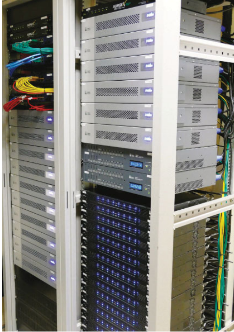
The BOH electrical room houses the racked D-Mitri processing platform
