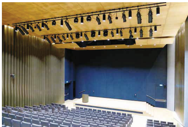
EAS had to install an L-C-R speaker solution and two lighting bars overhead
