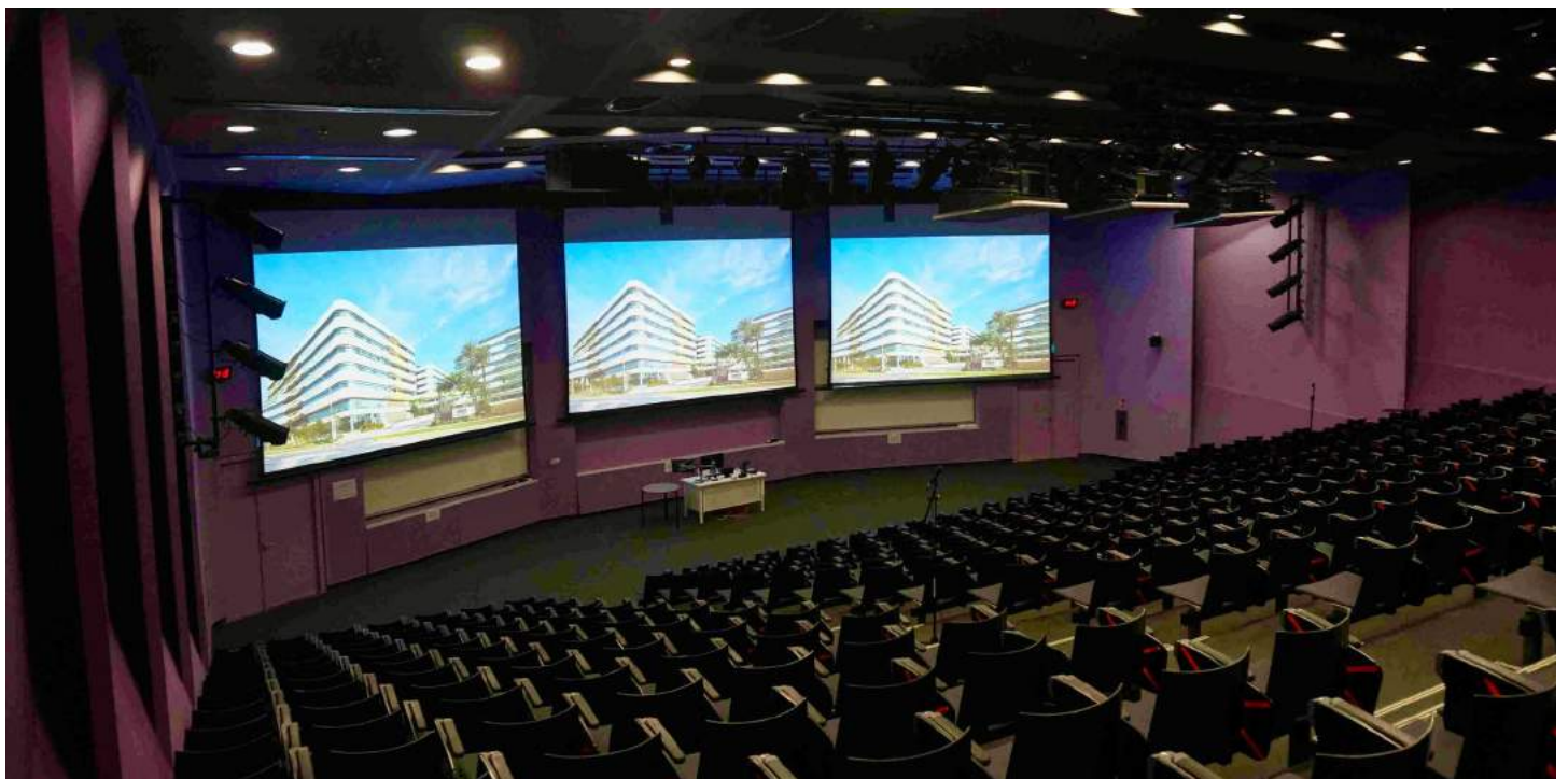
3 units of Epson EB-L20000UNL – 20,000 lumens, WUXGA,3LCD laser projectors are installed at the Lecture Theatre 1
