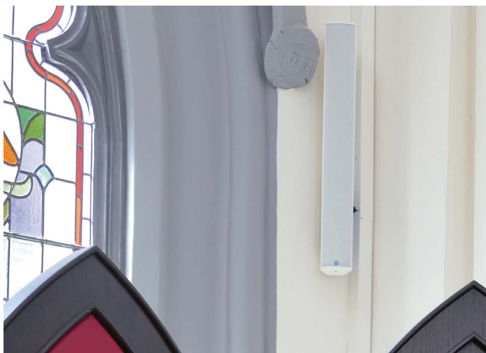
Smaller DC12/2 digital directivity control columns serve the naves
