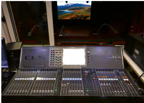
A Yamaha CL5 is located in the smaller auditorium’s control room
